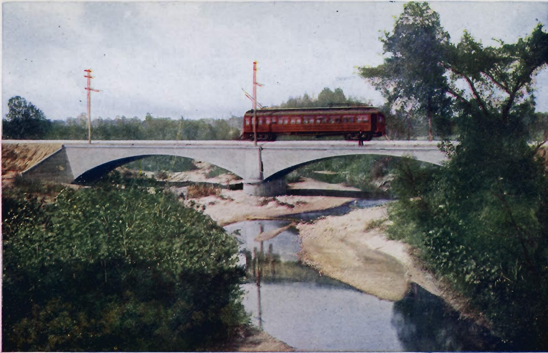
CARTERSBURG BRIDGE OVER WHITE LICK CREEK, CARTERSBURG, INDIANA Twin spans of 90 feet. Roadway 22 feet. Footings in clay with tie-plate. For the Terre Haute, Indianapolis and Eastern Traction Company, Indianapolis, Indiana, 1907. Photograph taken from Penna. R. R. Bridge since destroyed by protruding load on car striking steel trusses.
