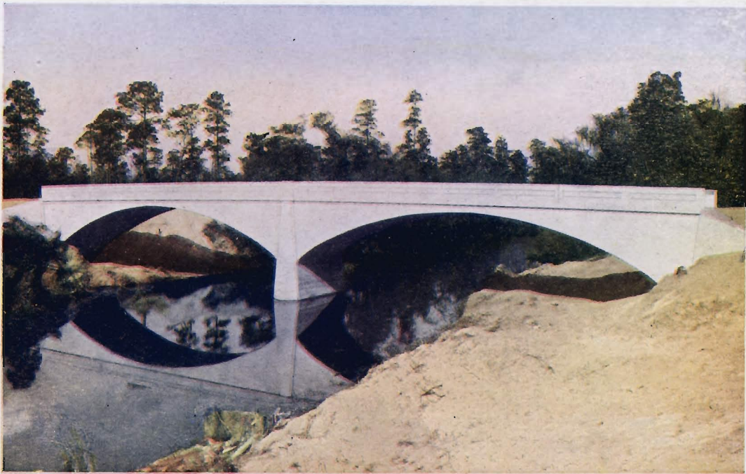
LITTLE RIVER BRIDGE, COLQUITT AND COOK COUNTIES, GEORGIA Twin spans of 70 feet each. Roadway 16 feet. Footings on marl. For the Boards of Commissioners of Colquitt and Cook Counties, Georgia, 1922.
